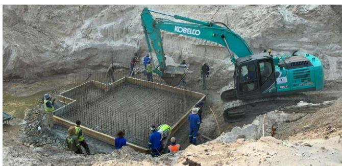
Construction of a sewer pump station in the Katima Mulilo project area.
