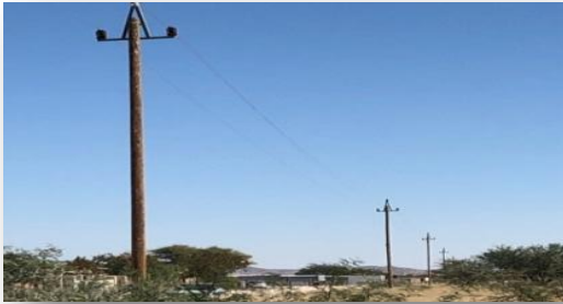
Figure 7: Electricity Poles and Streetlight on Portion 5
