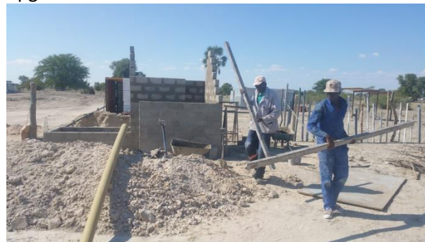
Reconstruction of an Okakedi pit latrine in Oshakati. More than 1300 of these well designed pit latrine models have been built in the 1990s and to date have made an immeasurable contribution to improved sanitation in the town’s informal settlements.
