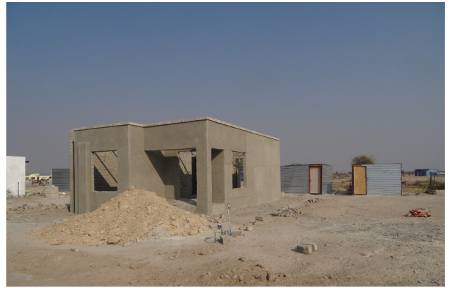
A house being built in Okahao with FNB loan, availed through the special FNB loan scheme for the clients of this programme
