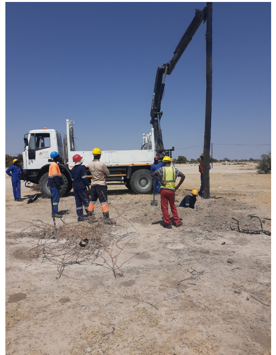
Right: Installation of the Electrical poles in Oshakati has commenced, the electrification is expected to be completed by the 30th of November 2021.
