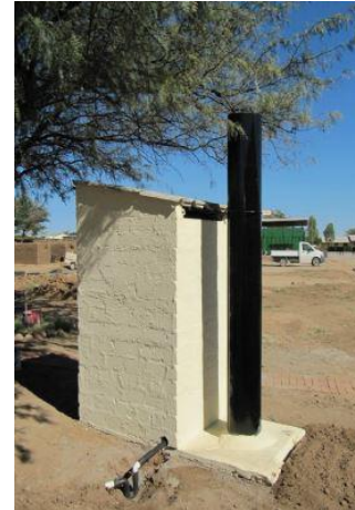
Professionally built VIP latrine, with extra big black ventilation pipe and urine diversion (Otjiwarongo; Ecosolutions, http://www.otjitoilet.org )
