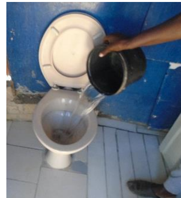
‘Normal’ toilet seat on pit latrine, floor with tiles, and used in combination with pour flush system (Havana, Windhoek)
