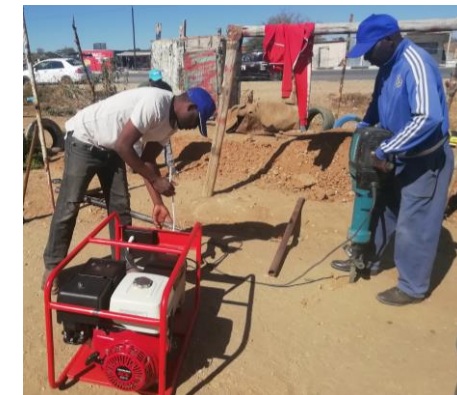
A jackhammer and generator are used to dig a latrine pit for a sanitation centre at a Windhoek kindergarten
